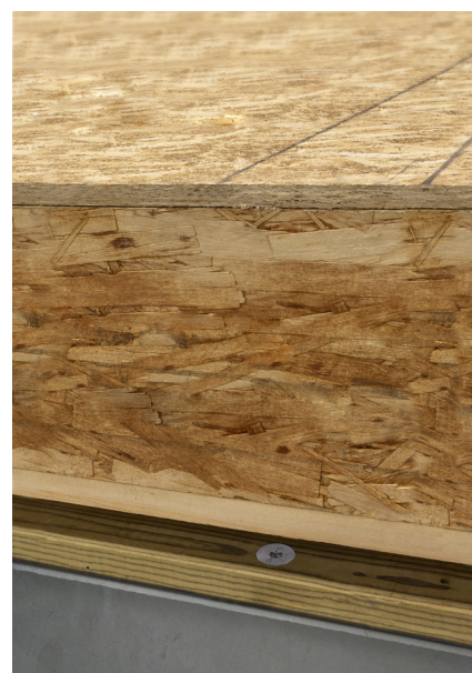
Modular floor panel installed on top of Titen HD Washer Head and sill plate.
